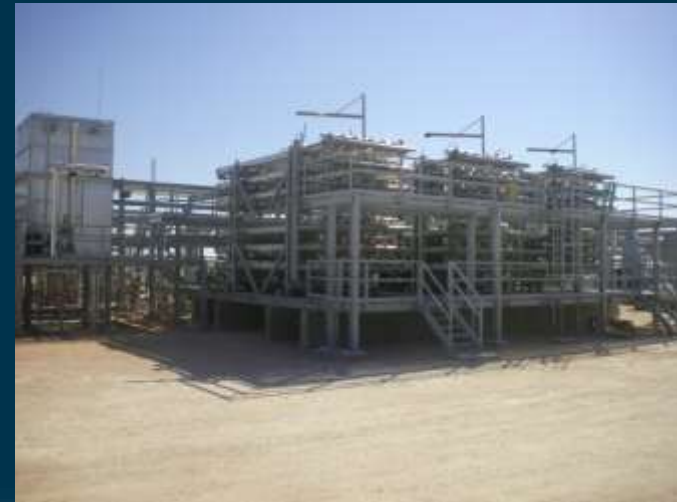
Whiting Petroleum (Wickett CO 2 Removal Facility) CO 2 Gas Membrane Equipment Valued at $3.5 Million West Texas, United States
