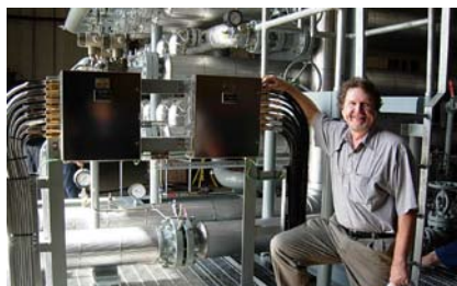
Projects I&E Manager Steve Keown with finished electrical equipment
