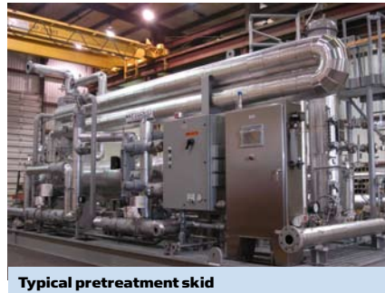
Typical pretreatment skid
